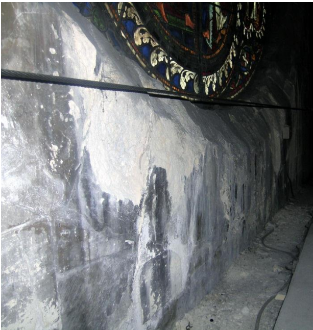
Fig.11: Water damage to stone cill
