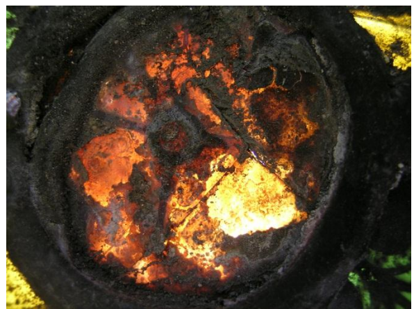
Fig.9: Corrosion damage – paint loss
