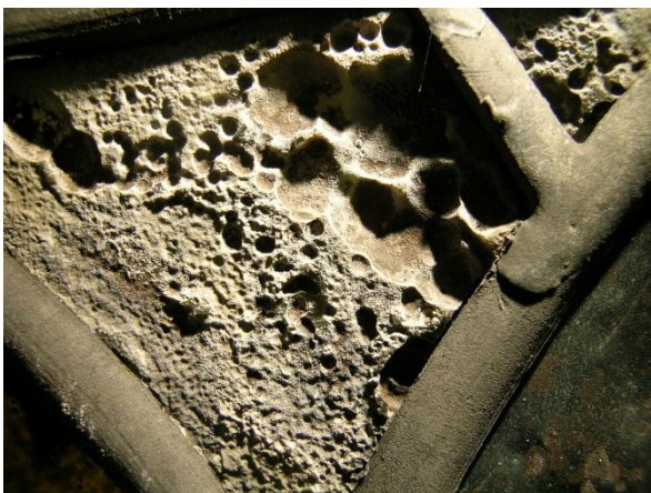
Fig.8: Corrosion damage – ‘pitting’
